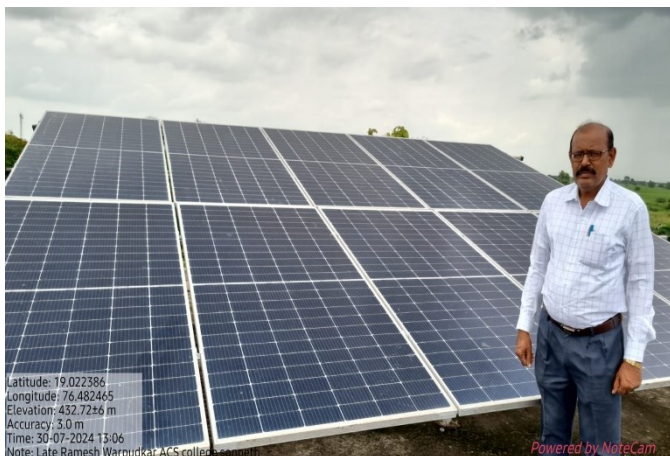
Solar Panels are installed in college
