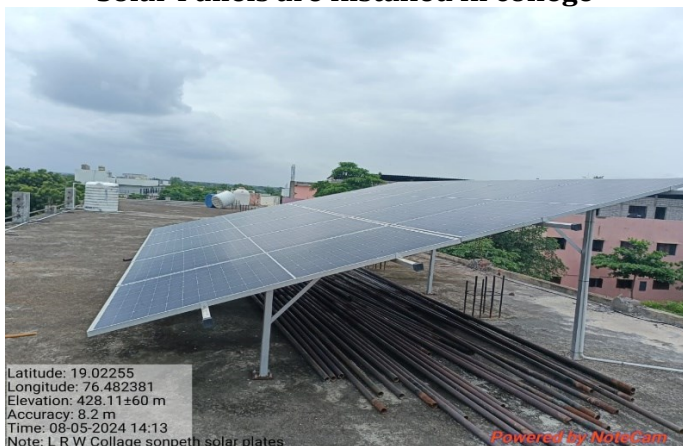
Solar Panels are installed in college
